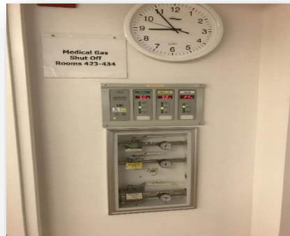
Unobstructed medical gas shutoff valve
