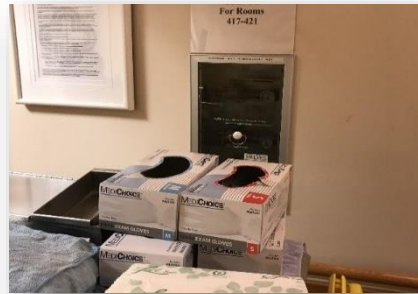
Blocked Medical Gas Shutoff Valve
